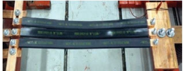
Before Short-circuit test
